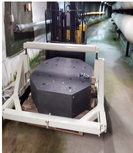
Figure 3: September 2014: the central granite block prepared for the installation phase; the weight of this central block is approximately 3 tons.
