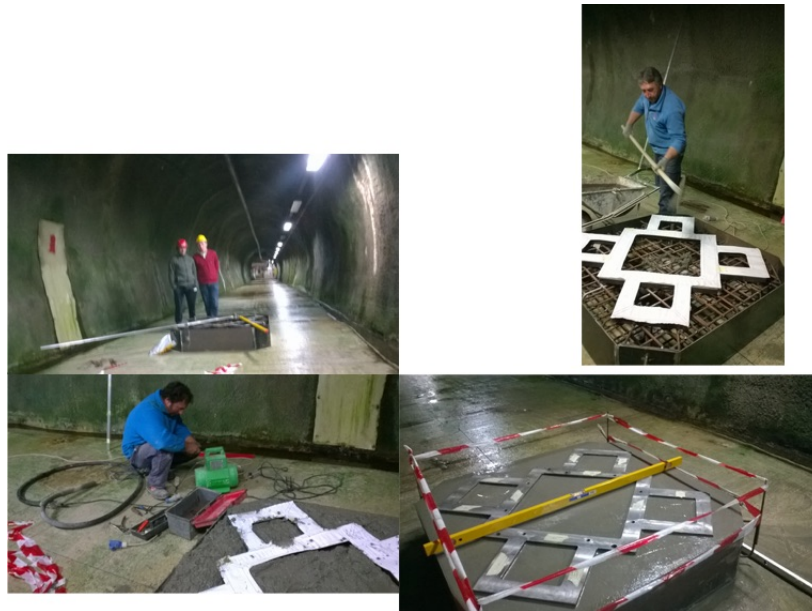
Figure 2: May 2014: the different phases of the installation of the reinforced concrete solid structure. The interface to attach the granite structure is well visible, this interface is immersed in the concrete, several rigid rods have been inserted in the underneath bedrock and in the concrete in order to well attach this structure to the bedrock itself.
