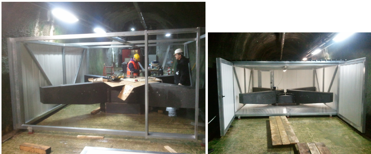
Figure 5: Left: Early phase of the installation of the box, Right: the box is complete
