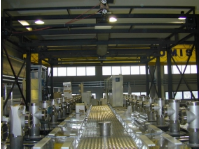
Figure 5: Top side of the T600 module during installation of the electronics racks.
