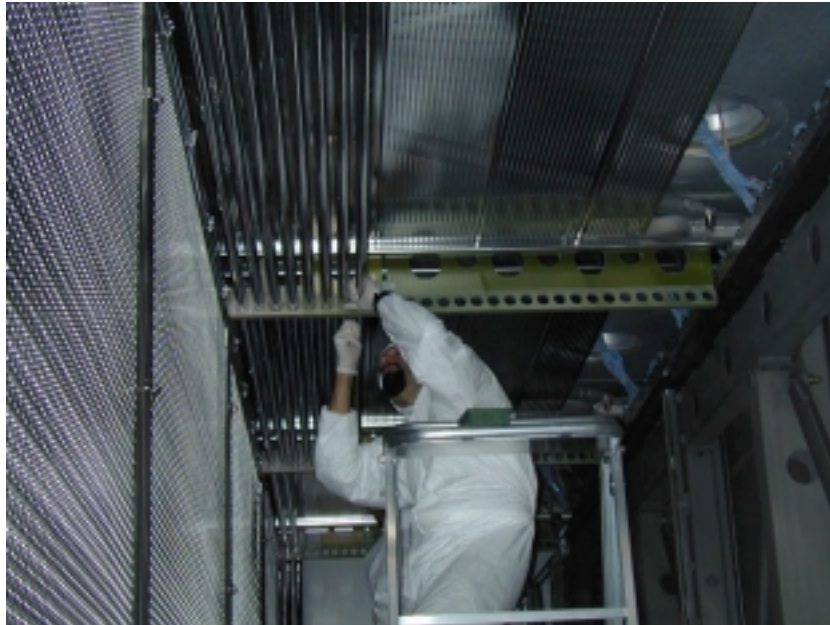
Figure 4: Picture of the electric field shaping electrodes (race tracks) mounting. In the middle of the cryostat the cathode is visible.
