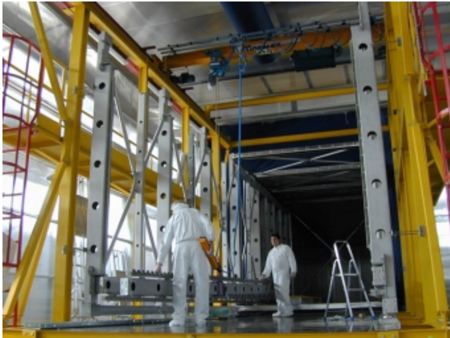
Figure 2: Picture of the (second third of the) sustaining structure mounting on the assembly island outside the cryostat. The first third is already inside the cryostat.
