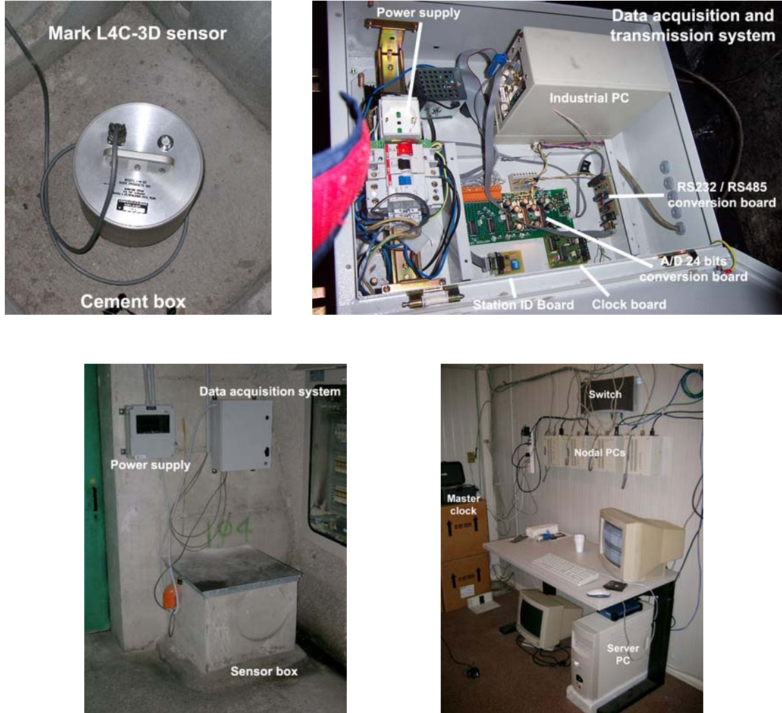
Figure 3: Underground Seismic Array components and control room.
