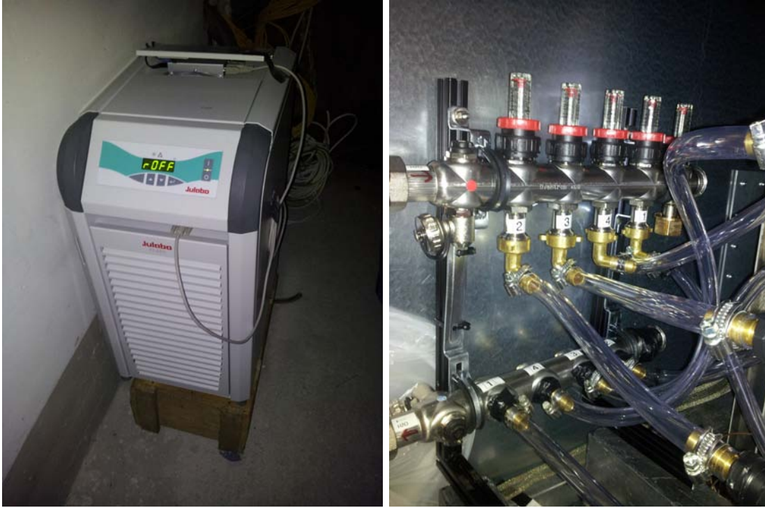
Figure 3: Left: Picture of the cooling device standing outside of the COBRA hut to dissipate the heat into the tunnel. Right: Picture of the preamplifier cooling system flow distributor supplying the cooling plates above the four preamplifier boxes. The flow in each sub-system can be adjusted individually, so that the uppermost one can be cooled the most, as it heats up most.
